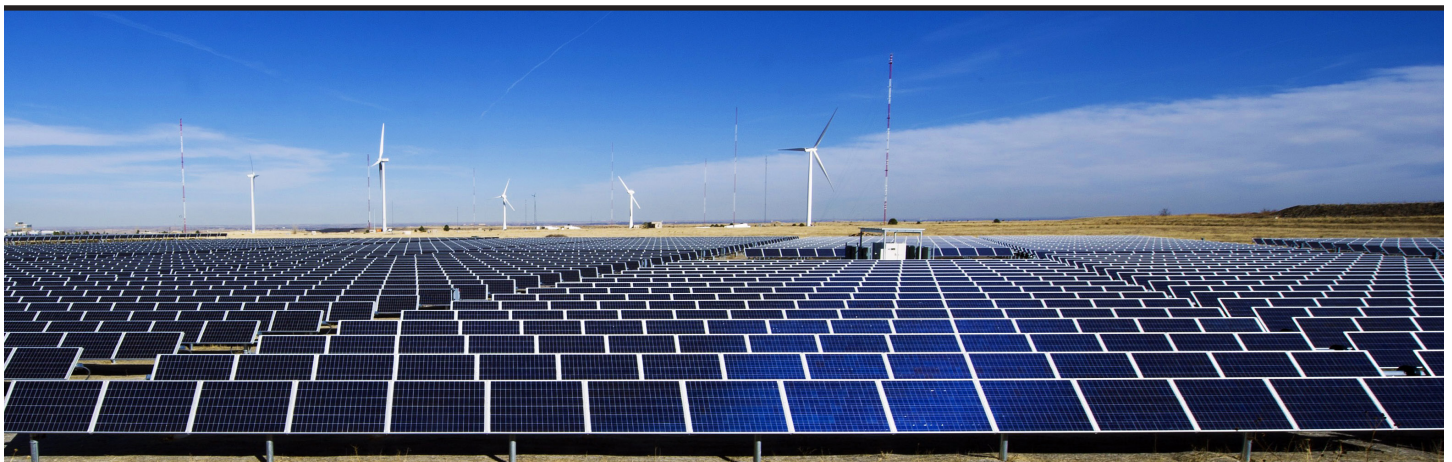
NREL’s photovoltaic array at the National Wind Technology Center near Boulder, Colorado. Source: US Department of Energy
